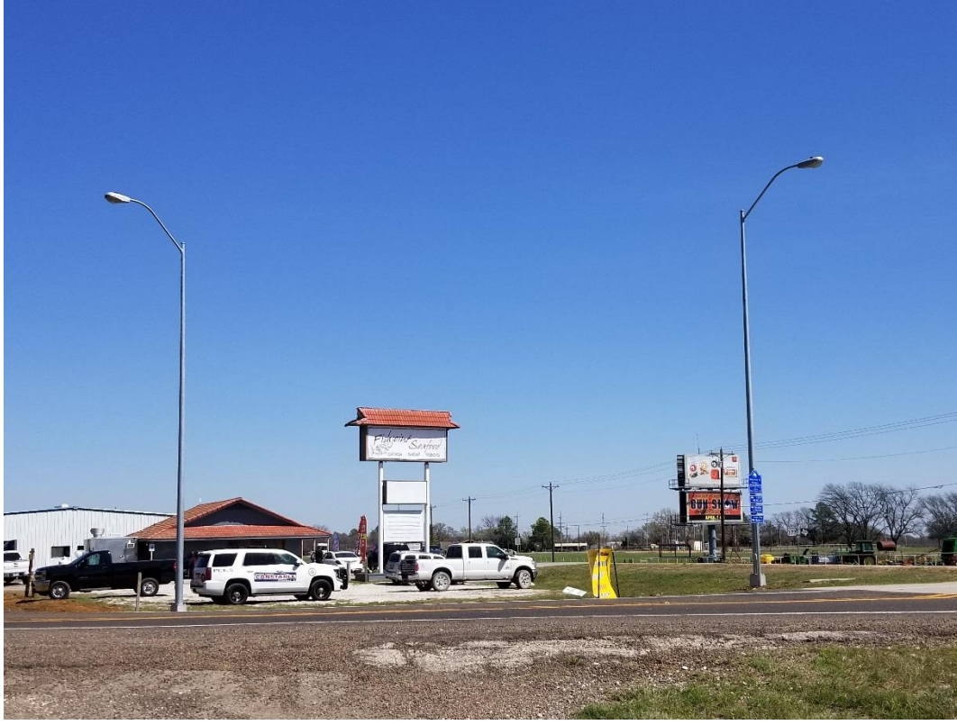
Street lights on the south end of Washington St.
